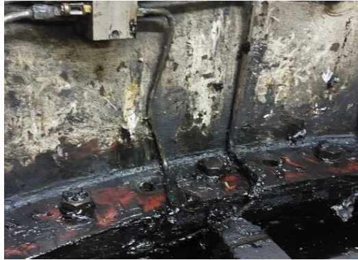
Gambar 1. Pengecekan Grease Point
