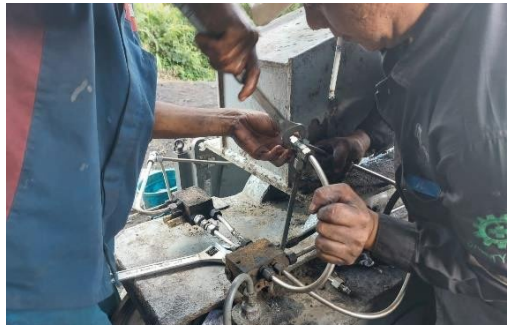
Gambar 3. Assembly Connector Distribution Line
